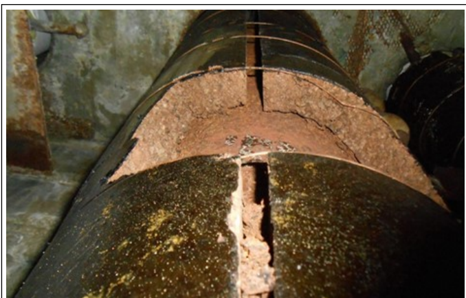
Fig.1. CUI in insulated carbon steel tube
